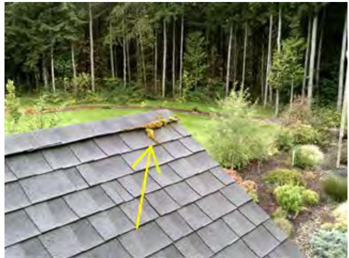
Photo 12-2 Moss on dormer ridge.
