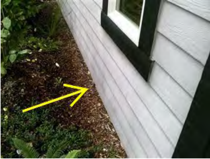
Photo 7-1 Earth siding contact at SE corner.
