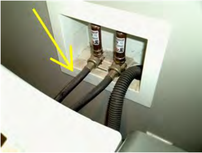
Photo 44-1 Rubber washer supply hoses.
