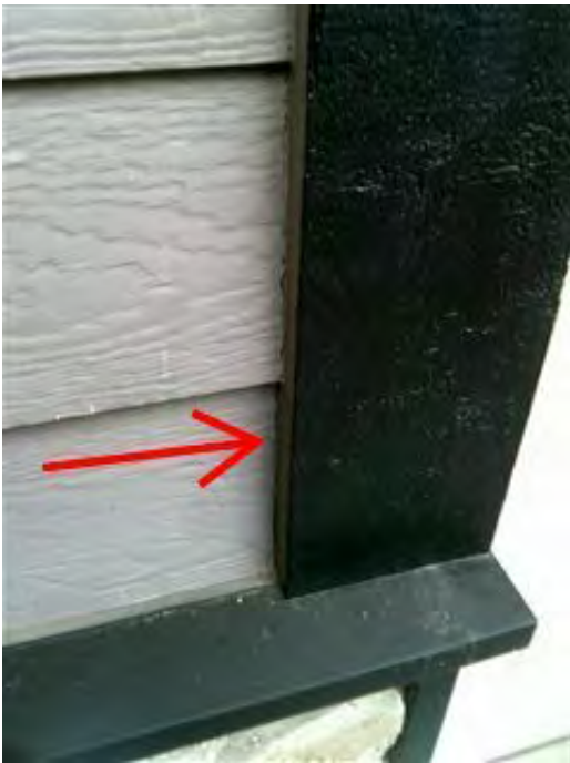
Photo 9-1 Deteriorated caulk at siding trim junction on garage.
