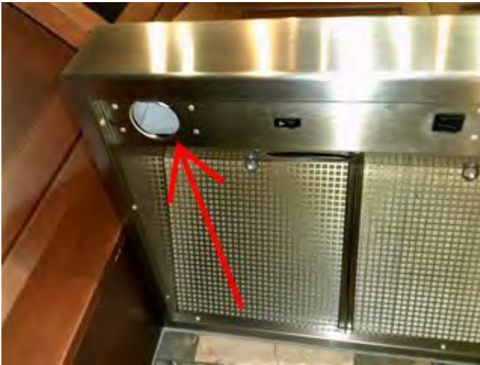
Photo 38-1 Missing bulb in cooktop hood.
