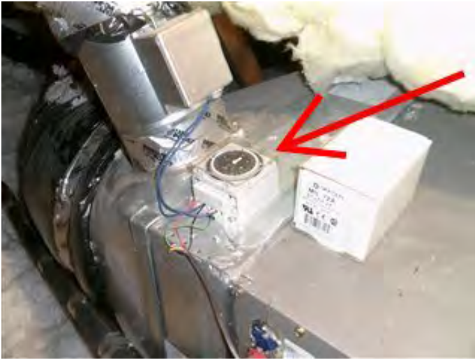
Photo 32-1 24 hour timer on furnace.
