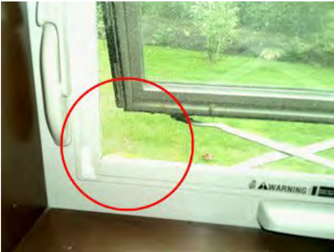
Photo 46-1 Damaged screen in bathroom #C toilet room.
