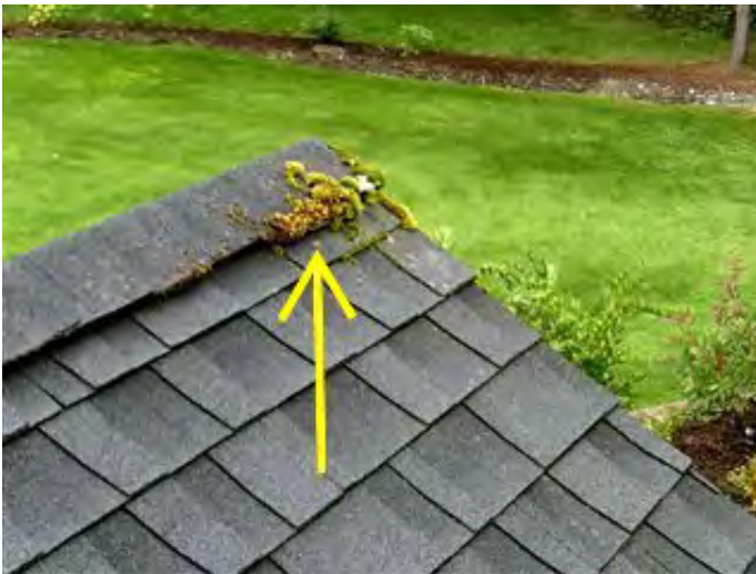
Photo 12-1 Moss on dormer ridge.
