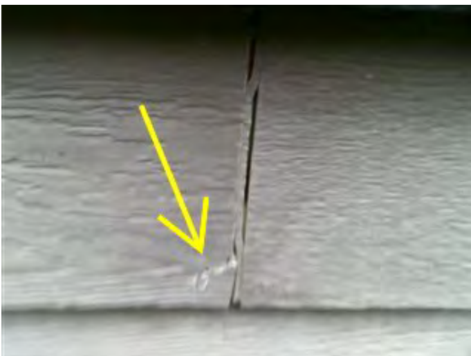
Photo 6-3 Damaged siding at butt joint on south side.
