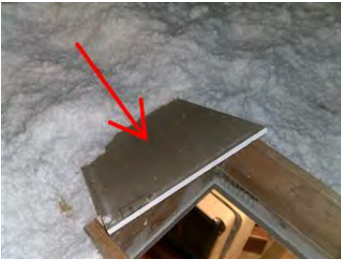
Photo 15-1 Missing insulation on hatch #B.
