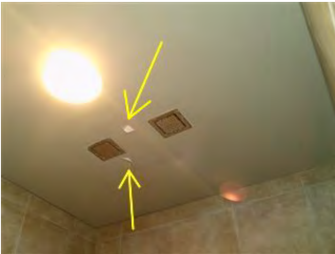
Photo 43-1 Damaged paint in shower #C ceiling.
