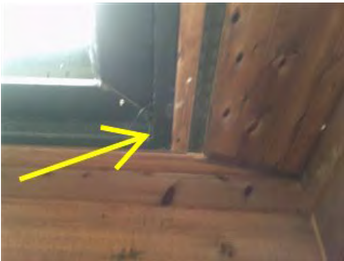
Photo 10-1 Gutter on rear porch leaking behind.
