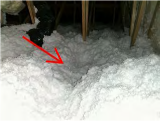
Photo 14-1 Uneven insulation in attic #A.
