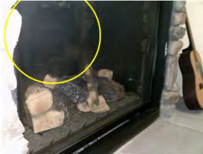
Photo 34-1 Fogging on living room fireplace.
