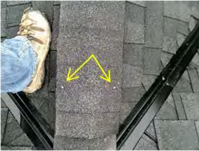
Photo 13-1 Exposed nails on ridge.
