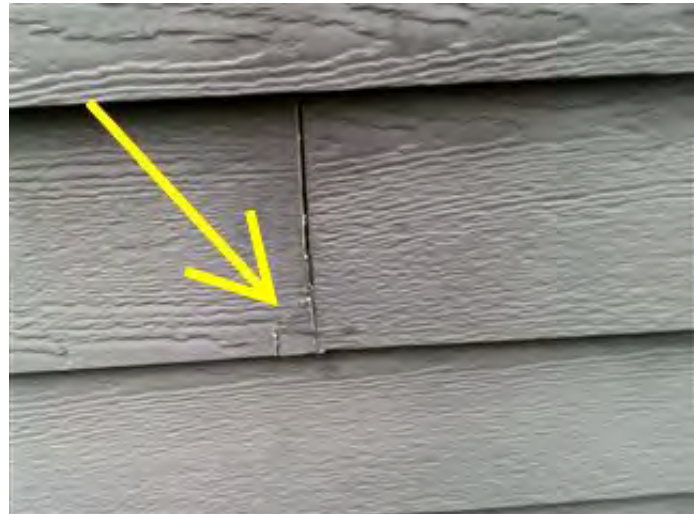
Photo 6-2 Damaged siding at butt joint on south side.
