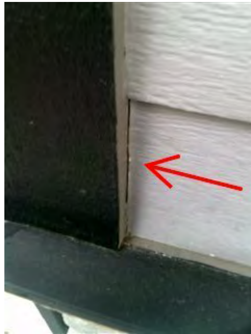
Photo 9-2 Deteriorated caulk at siding trim junction on garage.
