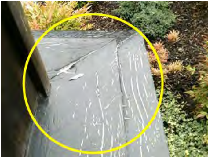
Photo 8-1 Deteriorated paint on pedestal cap.
