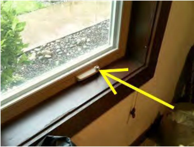
Photo 45-1 Missing window crank in SE bedroom.
