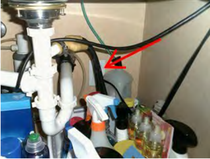
Photo 35-1 No air gap or high loop on dishwasher drain lines.
