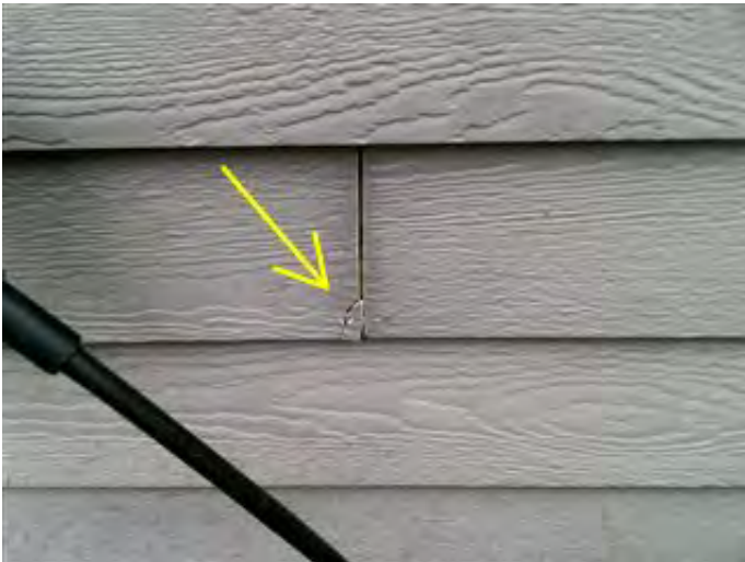
Photo 6-1 Damaged siding at butt joint on south side.
