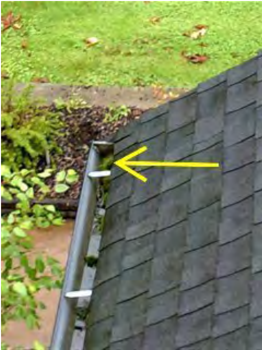
Photo 11-1 Debris in gutter at NE corner.
