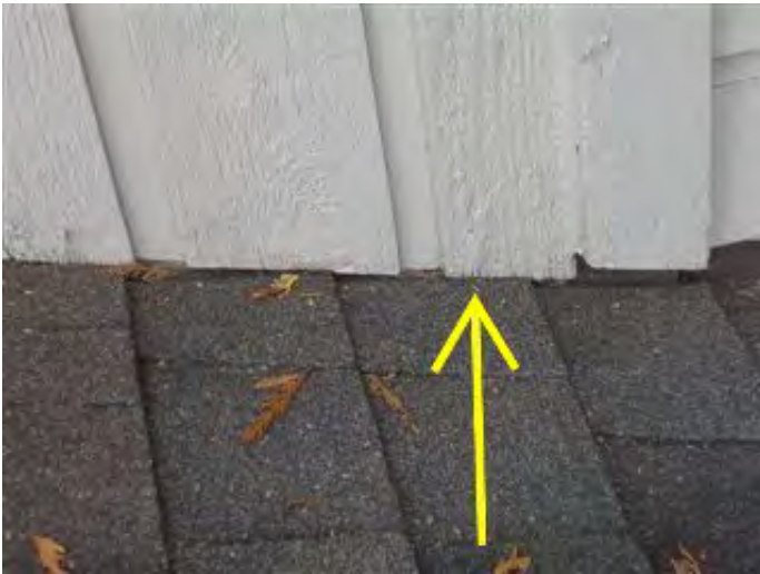
Photo 18-3 Siding in contact with roof cover over garage.
