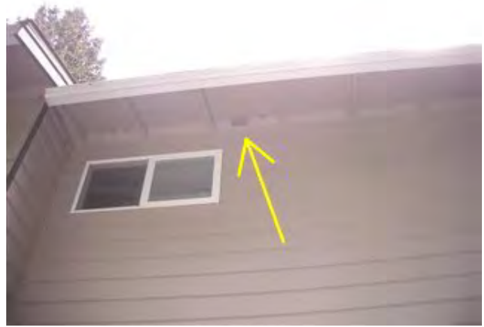
Photo 12-2 Damaged bird block on south side.
