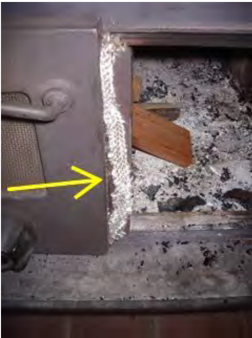
Photo 51-1 Deteriorated gasket on stove doors.
