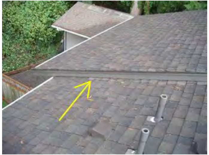
Photo 18-2 Trim in contact with roof covering.
