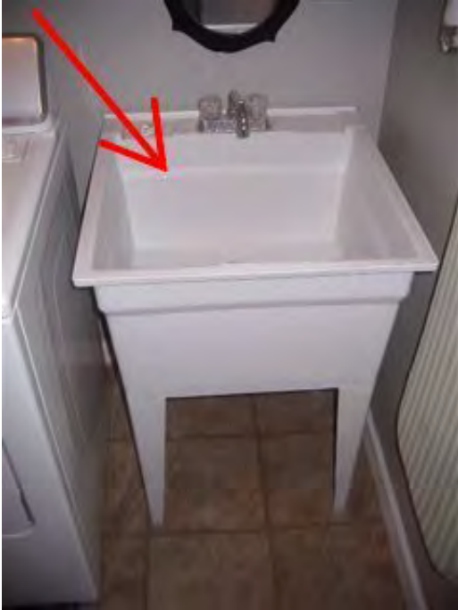
Photo 66-1 Laundry sink was loose.
