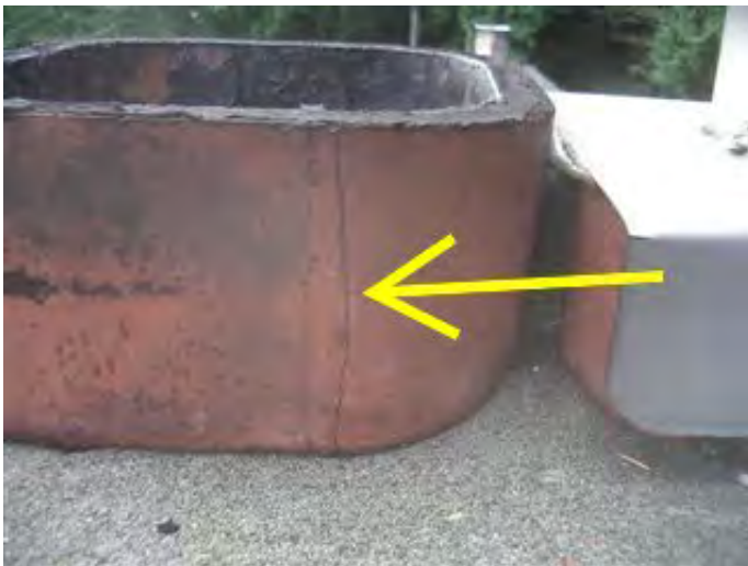
Photo 45-1 Crack in flue tile.
