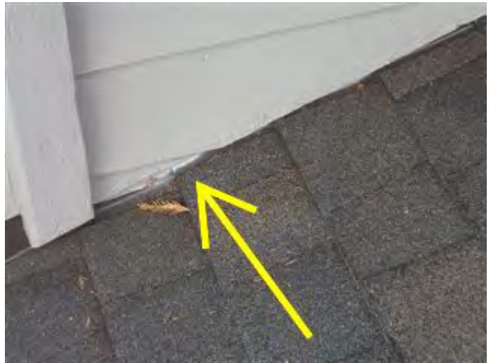
Photo 18-4 Siding in contact with roof cover over garage.
