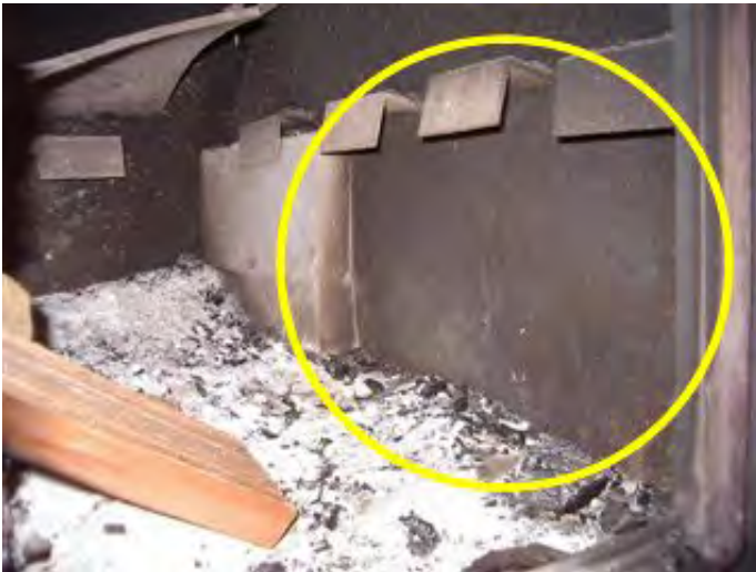
Photo 52-1 Missing fire bricks.
