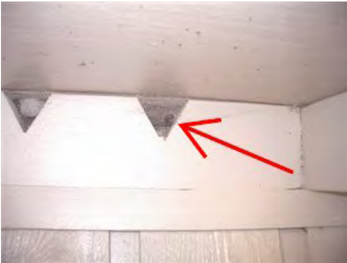
Photo 22-1 Damaged soffit vent screen over garage.
