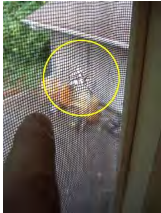
Photo 69-2 Damaged screen in master bedroom.
