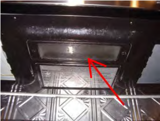
Photo 62-1 Exhaust hood light was inoperable.
