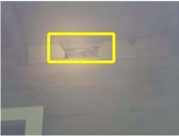
Photo 12-1 Damaged bird block on south side.
