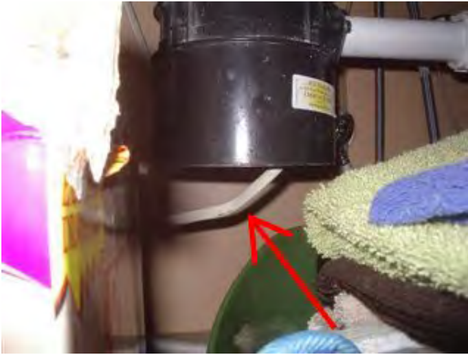
Photo 56-1 Non metallic sheathed wire to disposal.
