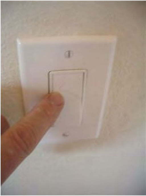
Photo 34-1 Cracked switch in NW bedroom.
