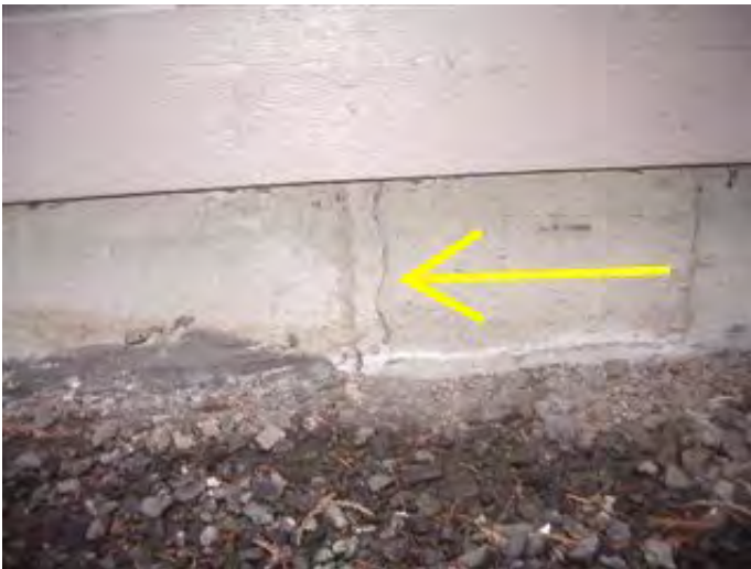
Photo 13-1 Minor crack in foundation on north side.
