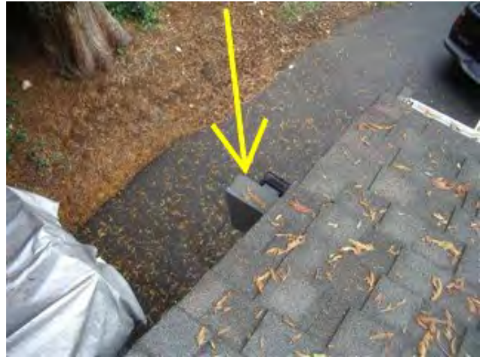
Photo 20-2 Exposed beam missing flashing.
