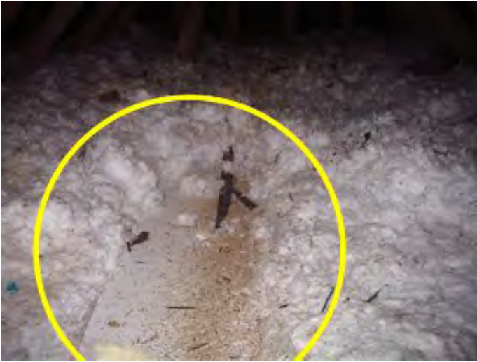
Photo 23-1 Uneven insulation in attic.
