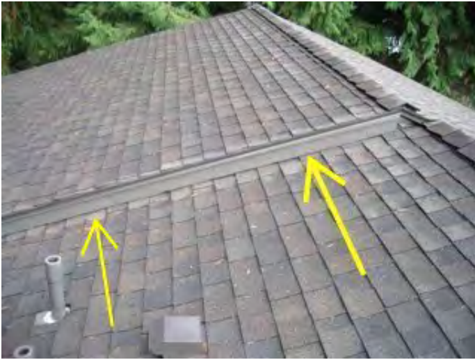
Photo 18-1 Trim in contact with roof covering.
