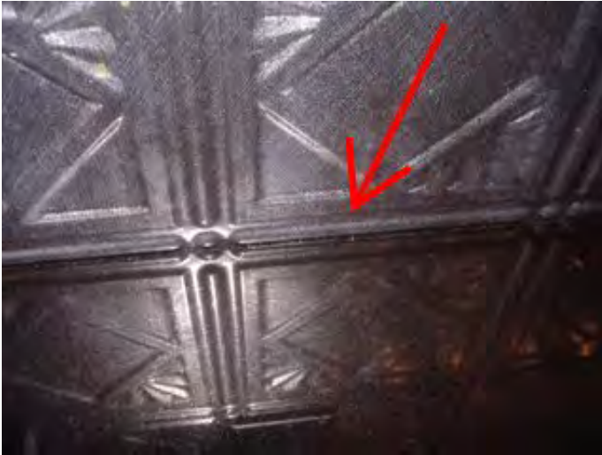
Photo 61-1 No caulk at backsplash.
