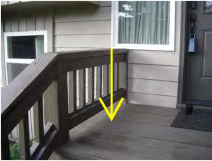
Photo 4-1 Entry railing too short.
