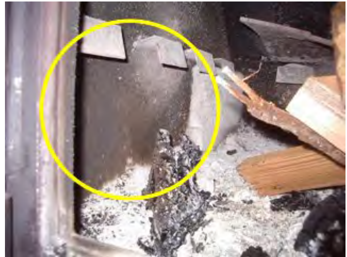
Photo 52-2 Missing fire bricks.
