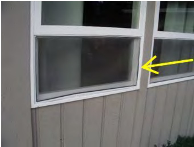
Photo 69-1 Damaged screen on basement window on north side.
