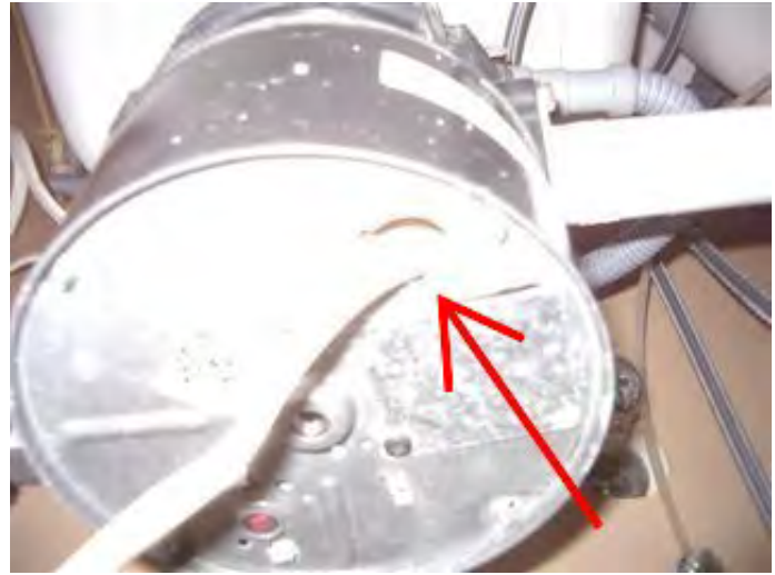
Photo 56-2 Missing bushing at disposal.
