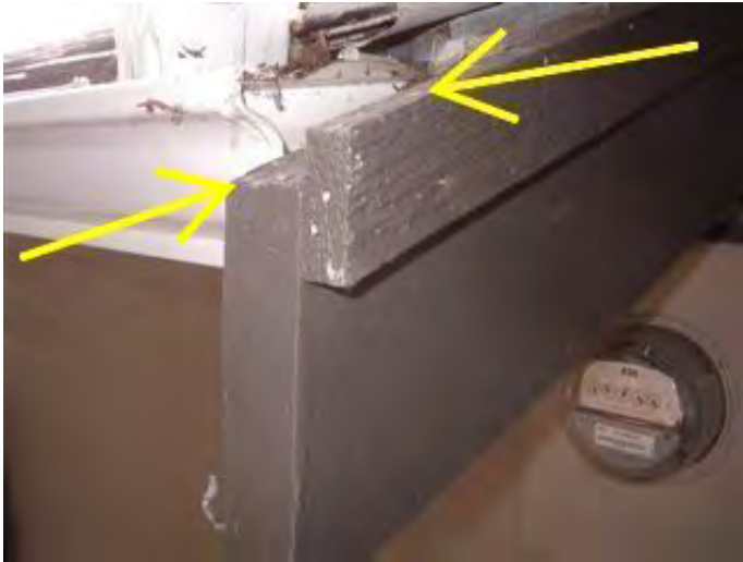
Photo 20-1 Exposed barge board on west side of garage.
