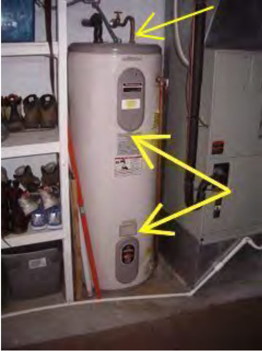
Photo 40-1 Missing seismic restraints.
