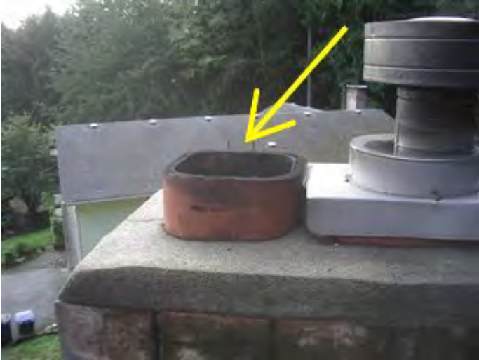
Photo 47-1 No spark screen or rain cap.
