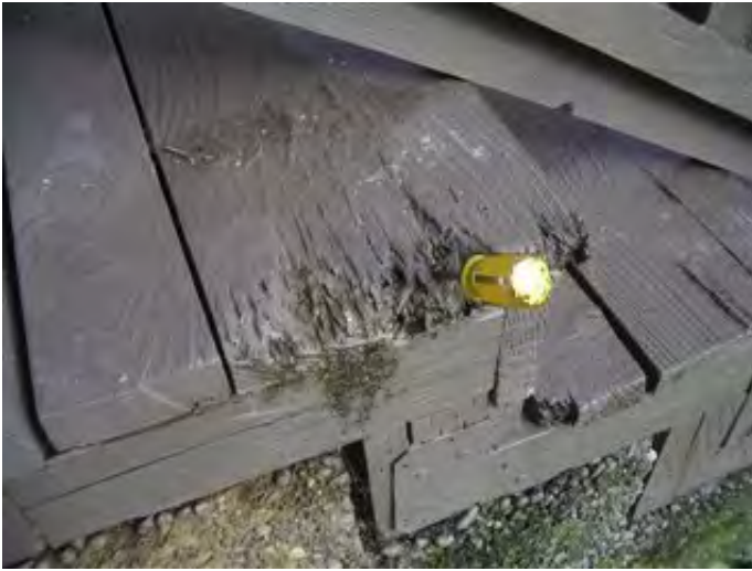
Photo 6-1 Rot in treads at entry.
