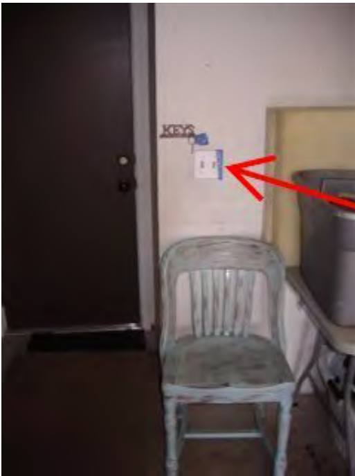
Photo 26-1 Control switch for automatic opener too low.
