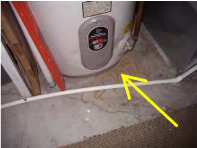
Photo 41-1 Missing insulating pad on concrete floor.
