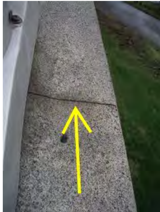
Photo 50-2 Crack in chimney crown.
