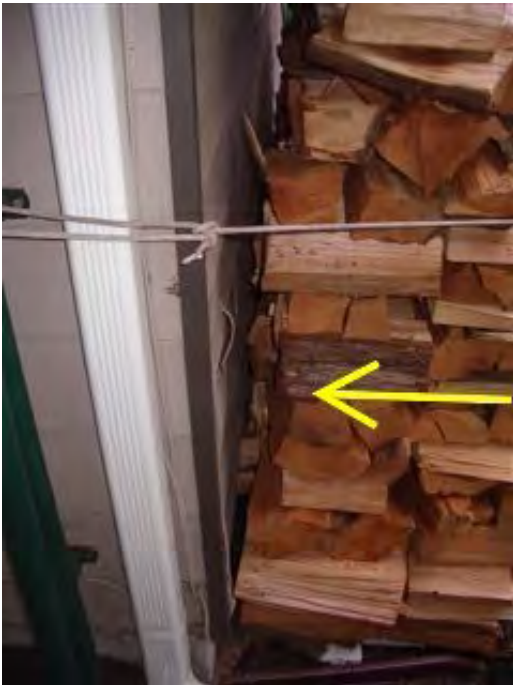
Photo 16-1 Firewood stacked next to house at SW corner.
