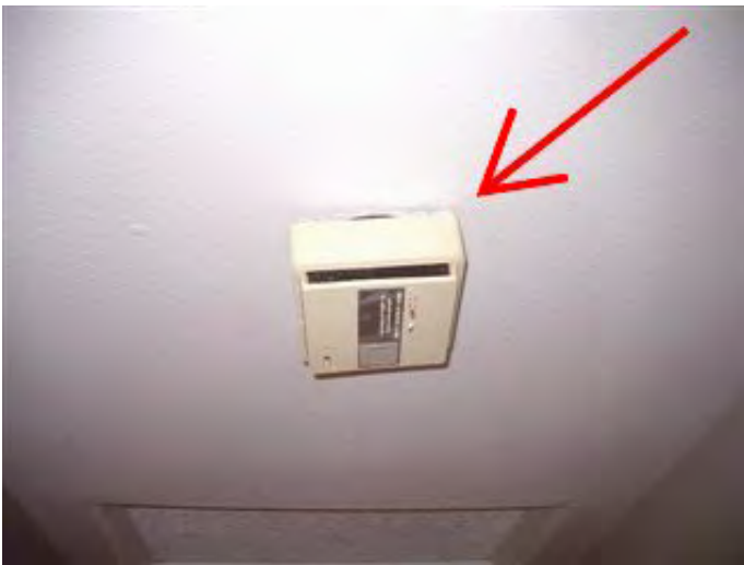
Photo 32-1 Older smoke alarm.
