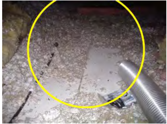
Photo 23-2 Uneven insulation in attic.
