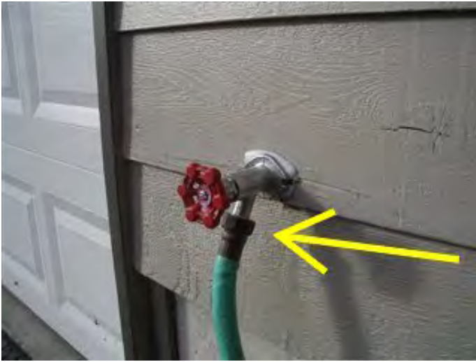
Photo 37-1 No backflow device.
