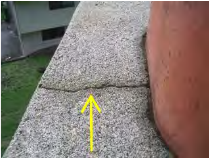
Photo 50-1 Crack in chimney crown.
