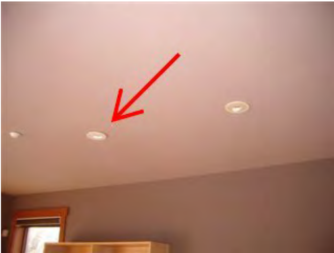
Photo 5-1 Loose light fixture over fireplace.
